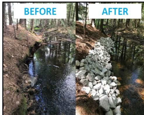
Riprap installed by 30MRWA's YCC stabilizes the soil and prevents it from washing into the stream.
