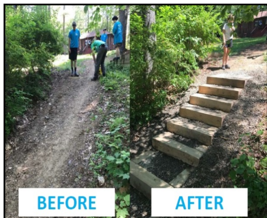
Infiltration steps installed by 30MRWA's YCC allow storm water to soak in, filtering it and reducing erosion.
